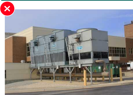
Exhibit 6-13. Unscreened mechanicals next to a building
